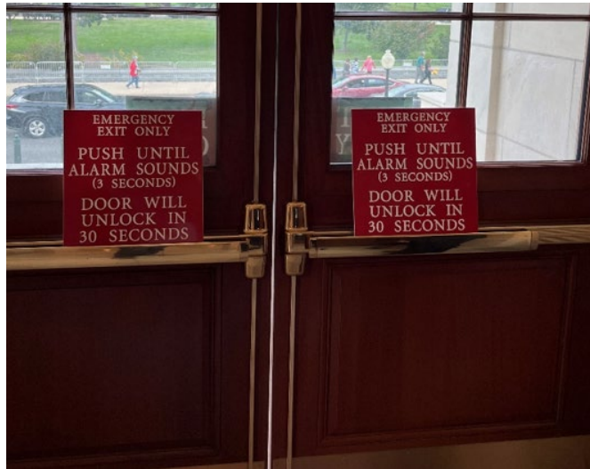
Image of Emergency Exit Signs atop Push Bar 22
