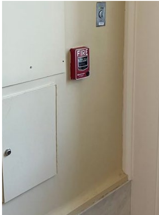
Image of Fire Alarm Station 27
